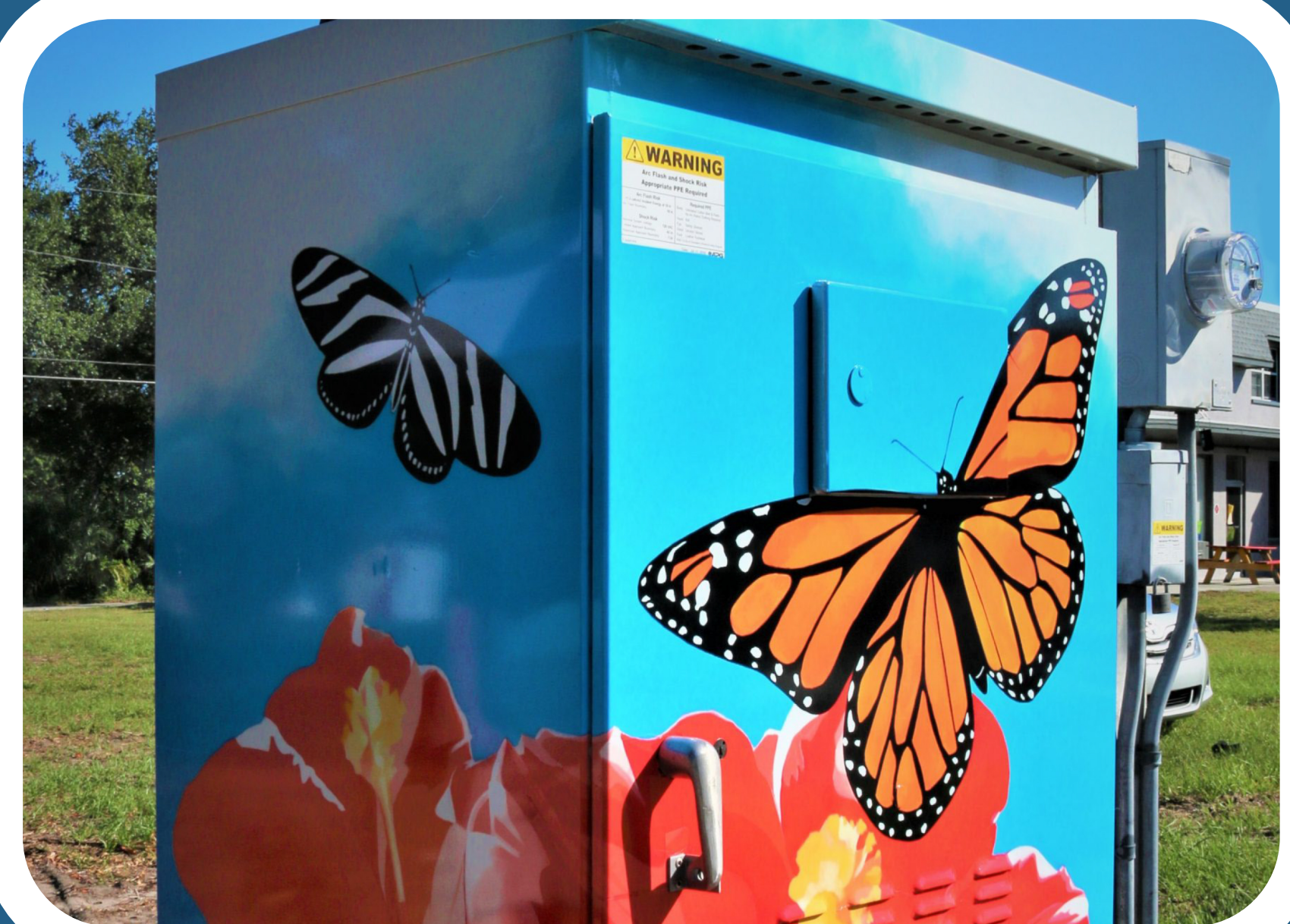
SIGNAL CABINET WRAP
