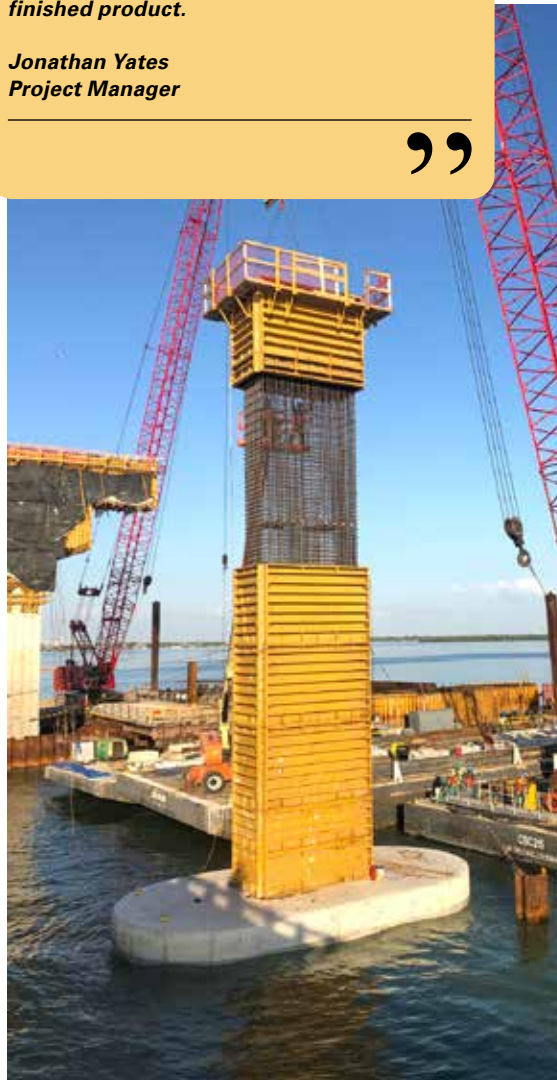
For the columns, AB chose the EFCO tieless PLATE GIRDER column forms.
